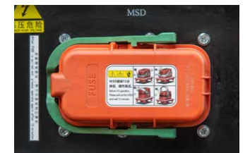
The MSD maintenance switch
